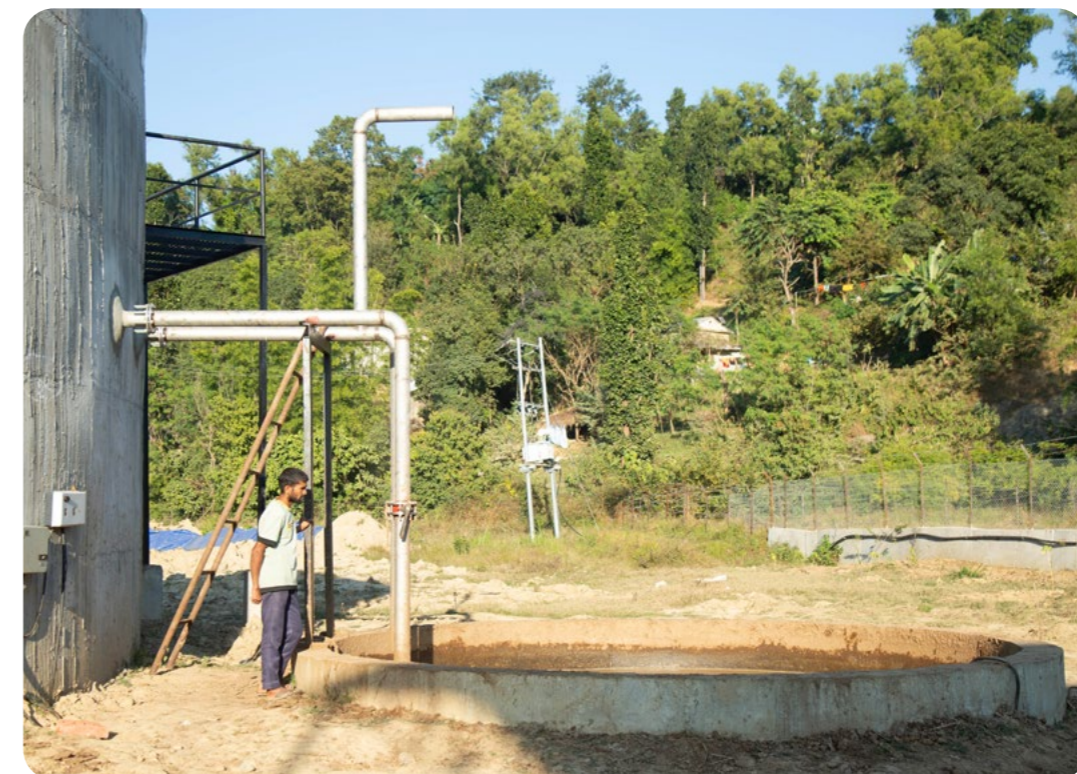
A worker stands over a churning pit of cow dung at a biogas plant in Surkhet, Nepal.
