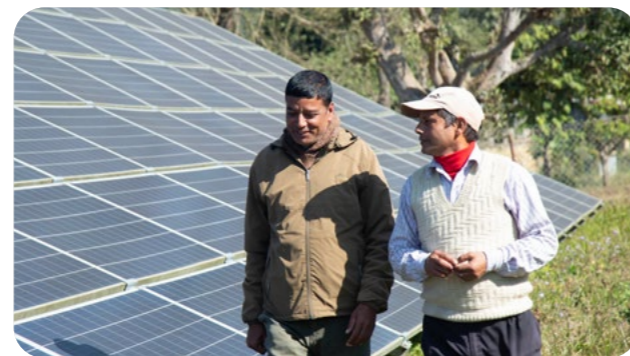
Engineers at a community solar installation in Gutu, Nepal.
