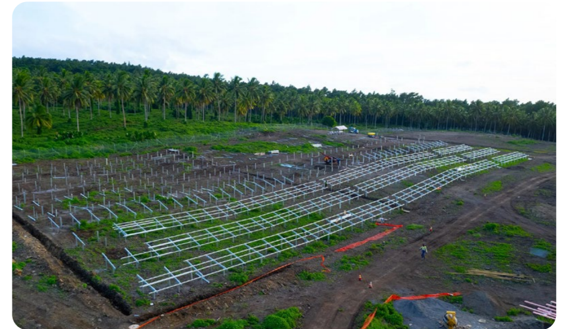
A solar installation and battery storage system being built on the island of Taveuni, Fiji
