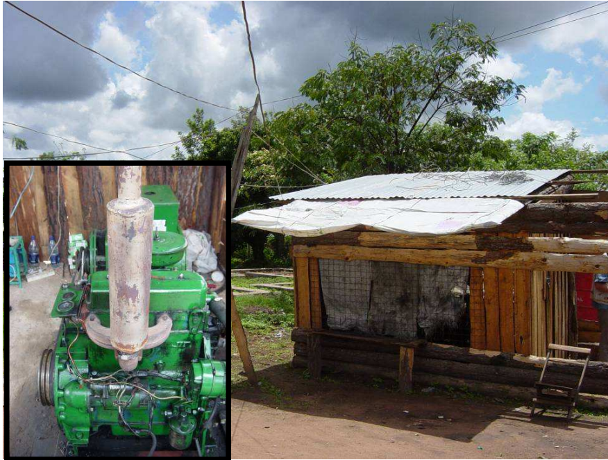
Figure 4: Generating house and distribution network for unlicensed power seller, inset shows the 54kW diesel generator enclosed in the wood building
