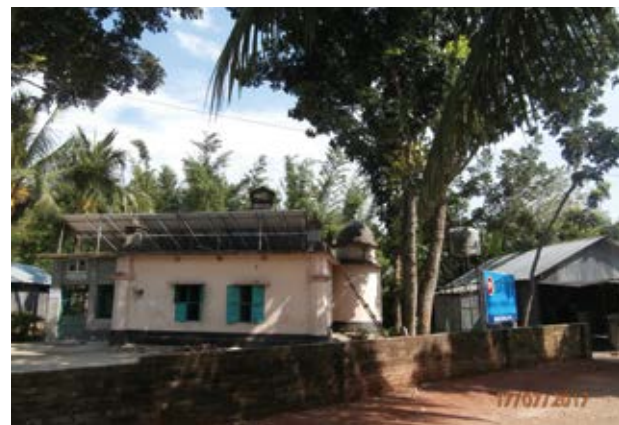
Left: One of the pilot installations in Kumargara. Staff reported that it gets much less hot inside the MCCs now that they are shaded by the solar panels. Credit: Enerplus
